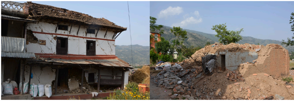
Fig. 7. Earthquake damages in Aalapot.
